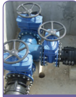
Martigues Power Plant, France, Marseille, AquaGrip
