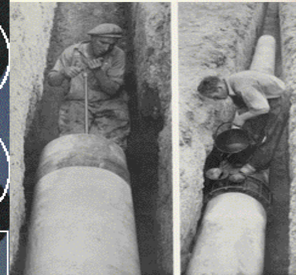
Left - Operator adjusting the coupler and having locking up pipe into position for turning the shaft. Right - Working between couplers to complete the inner connection. The shaft extends to the left side of right side pipe as it will fold to indicate when the coupler is in the required form.
