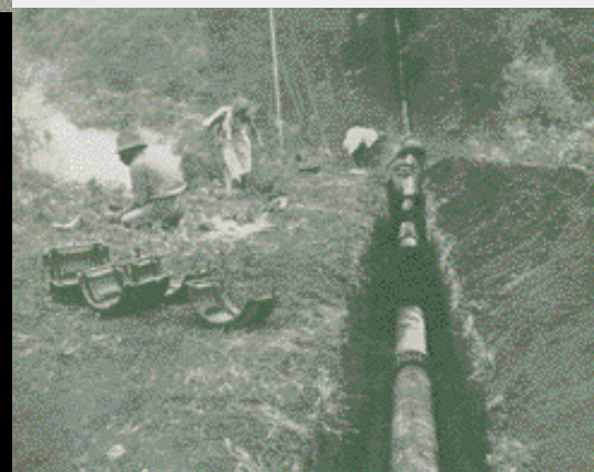
Some pipelines with Viking Johnson couplings
