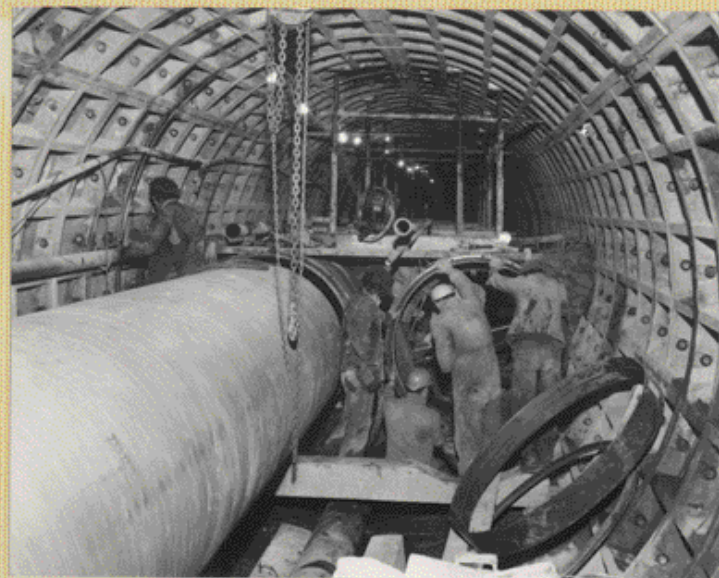
NORTHUMBRIA WATER AUTHORITY. Tyneside Interceptor Sewer June 1975. 55 1/2" V.I.C. on Redlands GRP Pipe
